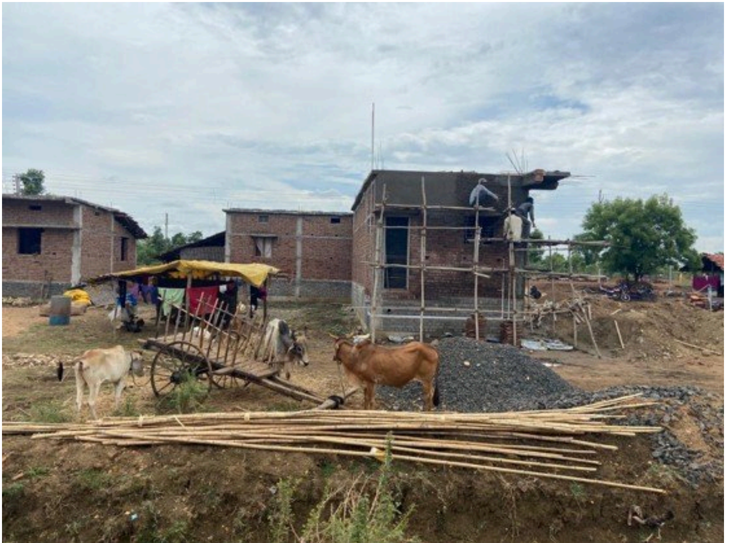
New Rantalodhi in the process of building at the relocation site after relocation from Tadoba-Andheri Tiger Reserve, Maharashtra, 2023. Photo by Prerna Singh Bindra.
