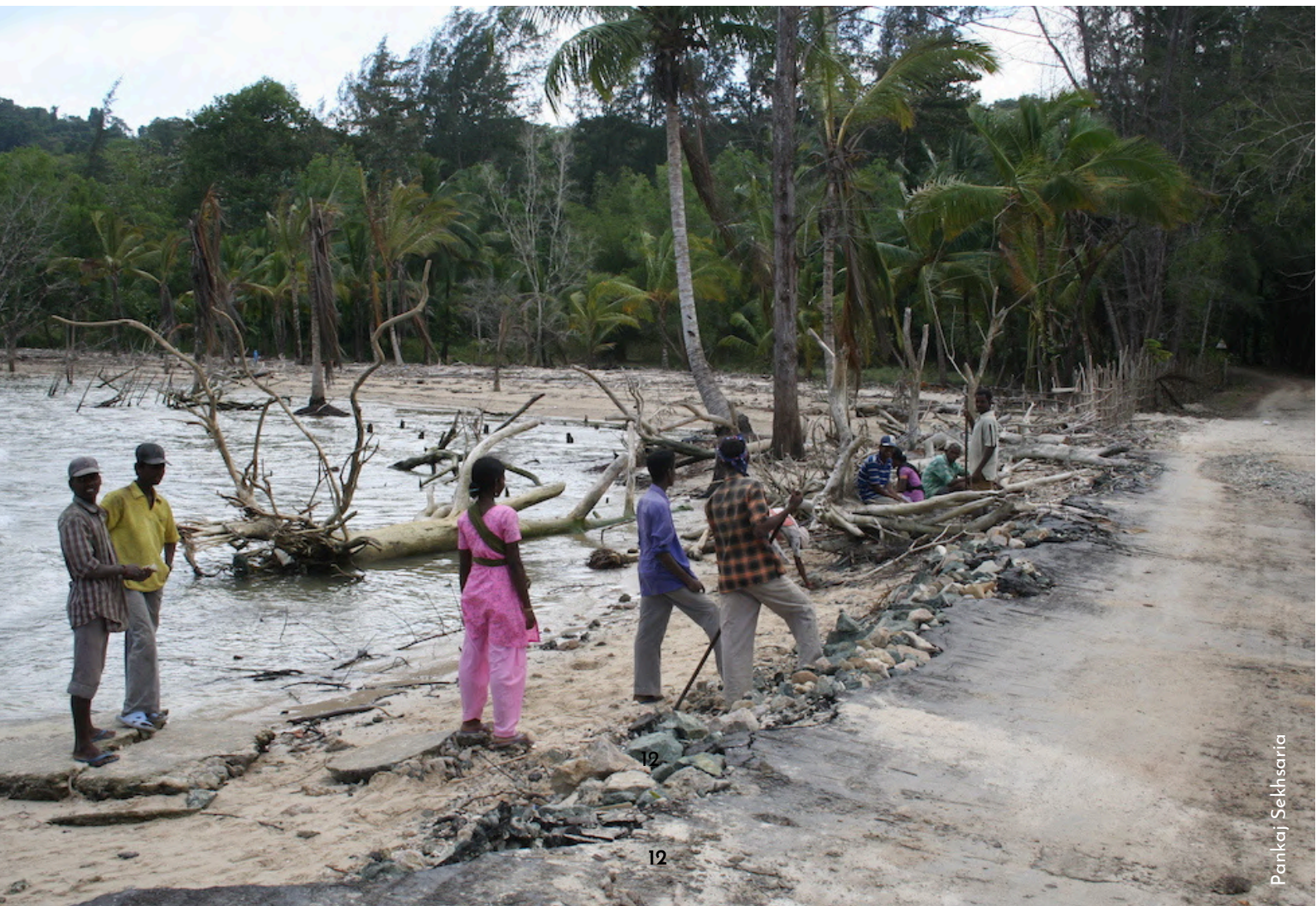
Working on the coastal road just outside Campbell Bay in 2006. It was washed out by the December 2004 earthquake and tsunami.
