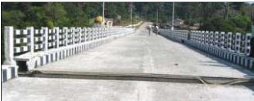
Figure 10b. Detail of the bridge deck showing lateral and vertical displacement due to shifting of the decks on their neoprene bearings (photo: Durgesh C. Rai).
