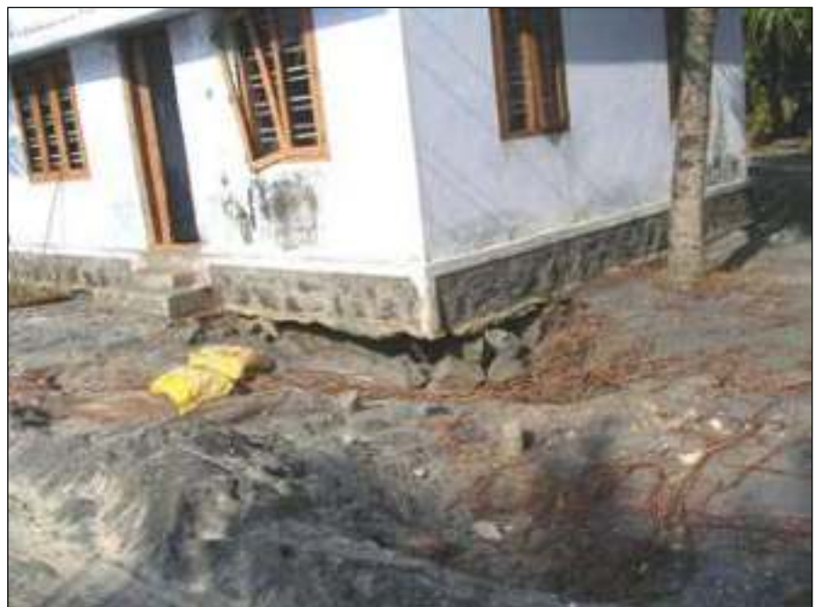
Figure 16. Scouring action at the base of houses due to returning wave of the tsunami in Kollam district in Kerala (photo: Alpa R. Sheth).
