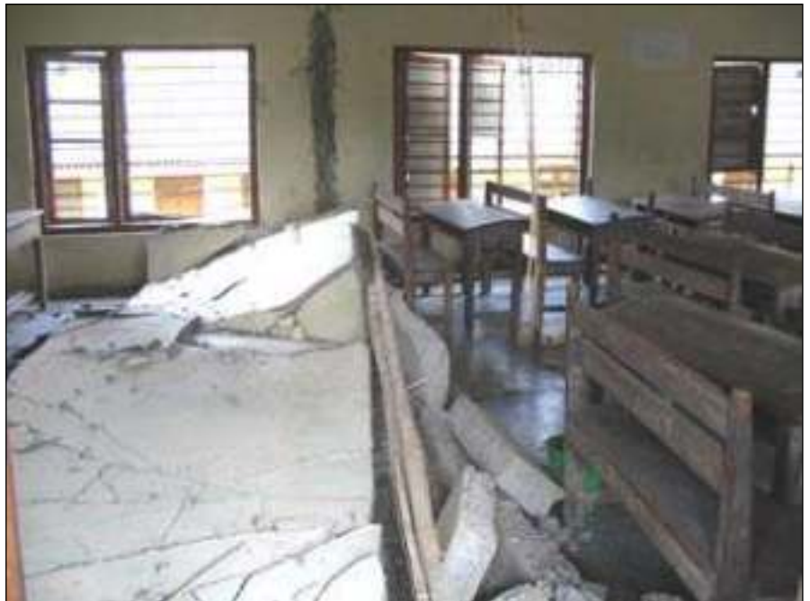
Figure 8. Slender masonry walls dislodged due to out-of-plane instability and poor or no connection to the surrounding structural elements (photo: Durgesh C. Rai).
