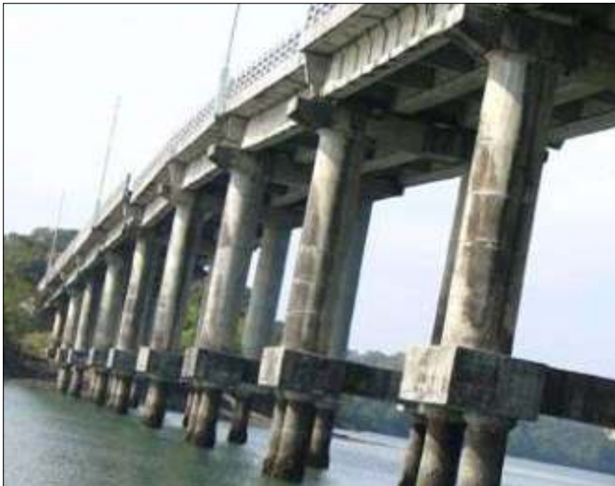
Figure 10a. Chengappa Bridge over Austen Strait was rendered dysfunctional by displacement of the middle spans (photo: Durgesh C. Rai).
