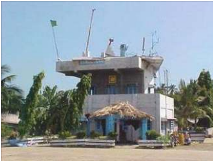
Figure 12a. Partial-collapse of the upper storey of the air traffic control tower at airport on Car Nicobar Island (photo: C.V.R. Murty).
