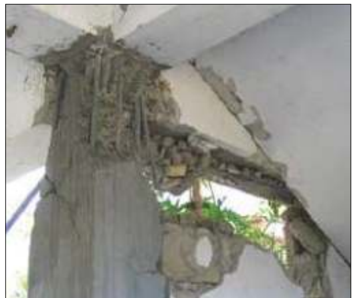
Figure 9b. Detail of column failure in the ground story (photo: Durgesh C. Rai).
