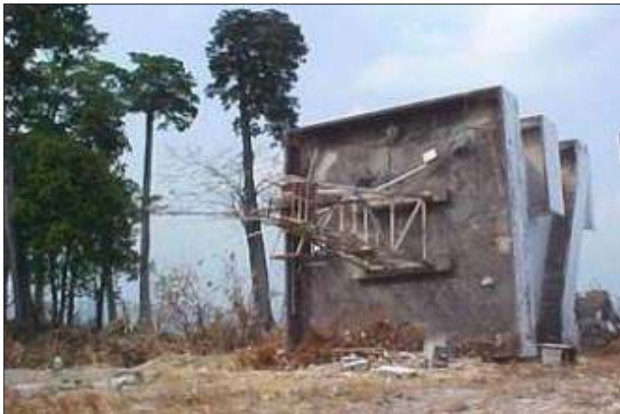
Figure 12b. Laterally toppled three-storey seaport traffic control tower at Hut Bay in Little Andaman Island (photo: Suresh R. Dash).
